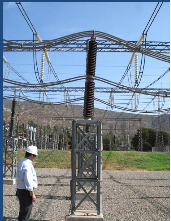
Electrical Substation, near Quillota, inclined Isolator
