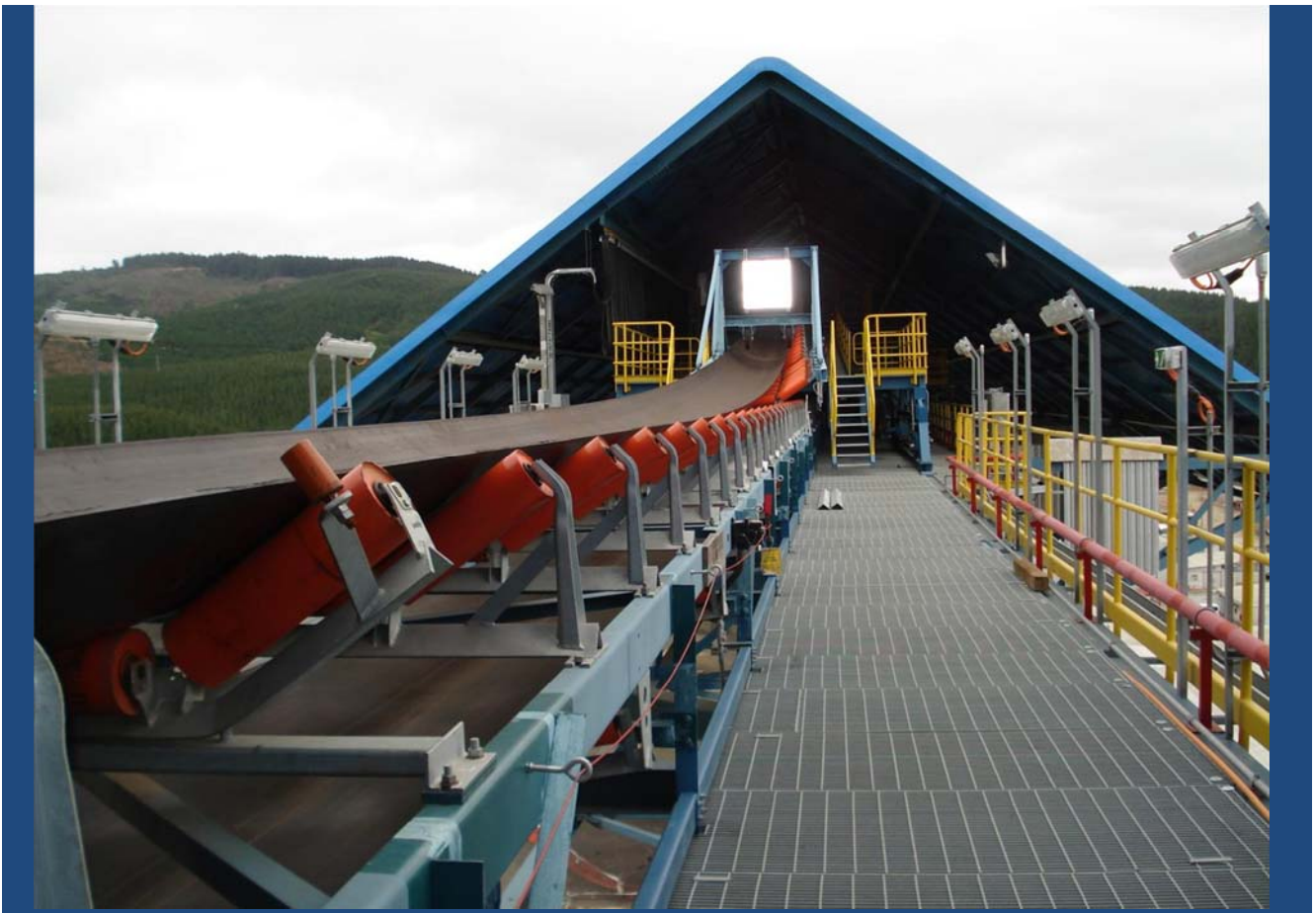
Correa Apilador de Carbón, Central Termo-eléctrica, Zona Coronel Conveyor for Coal Tripper, Coal Fired Power Station, near Coronel (under Construction)
