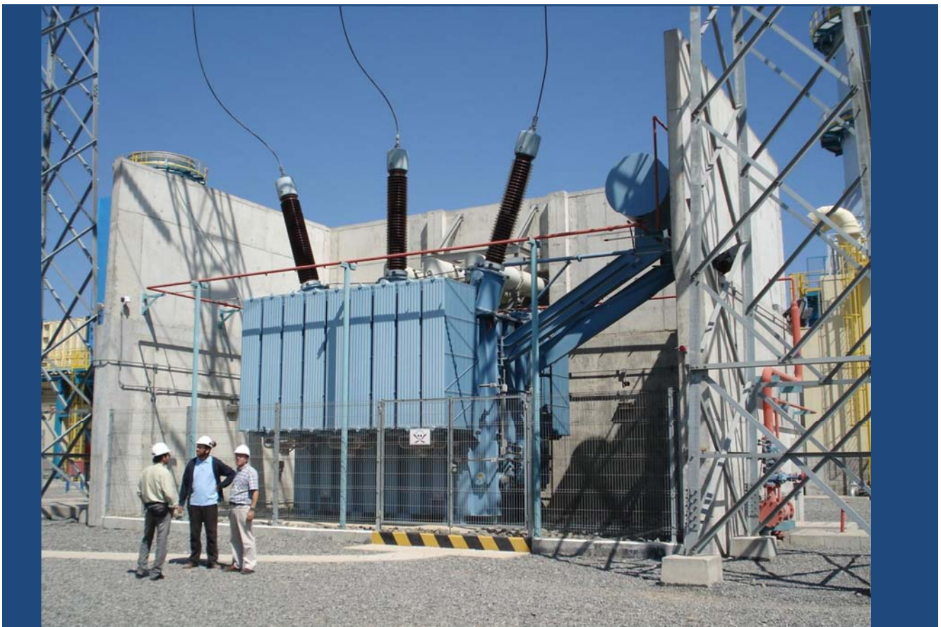
Transformador Principal, Central Termo-eléctrica, cercano a Codegua. Main Transformer, Diesel Fired Power Station , near Codegua
