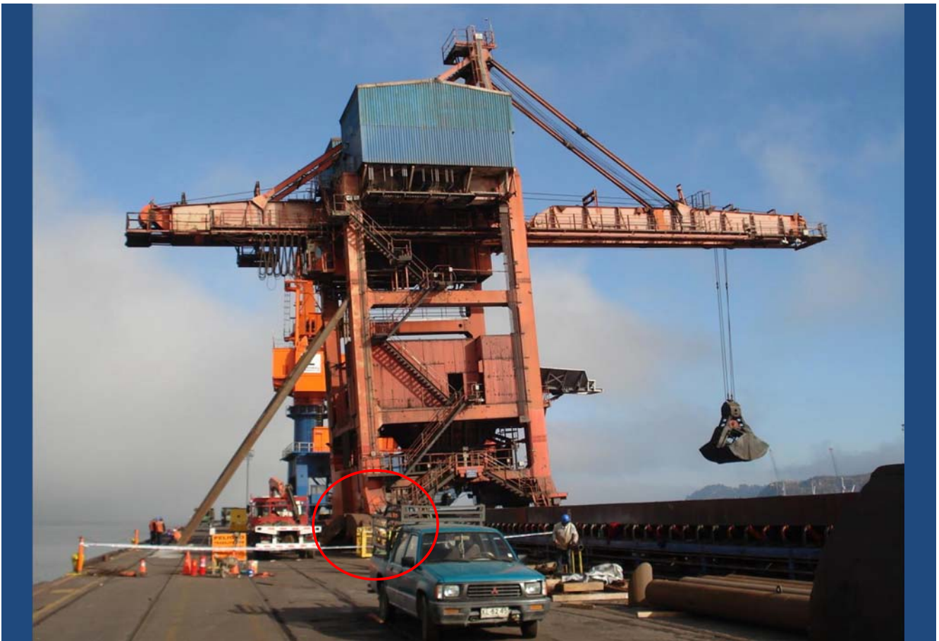
Huachipato, Large crane for Bulk cargo, Failure of columns at base (rails), due to overturning. Temporary diagonal support.
