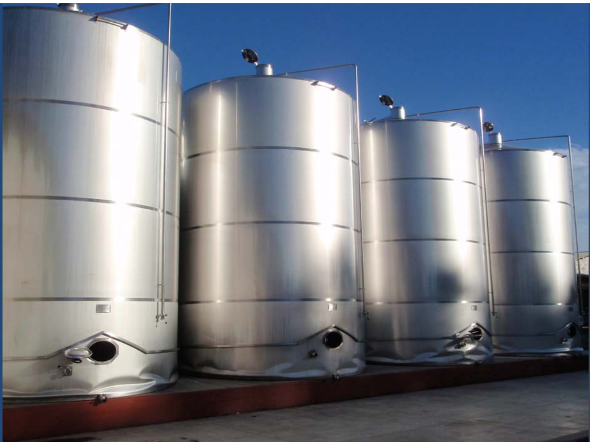
Falla Base Estanques de Acero Inoxidable para Almacenamiento de Vino. Cercano a Curicó. Failure at Base of Stainless Steel Storage Tanks, Winery near Curicó
