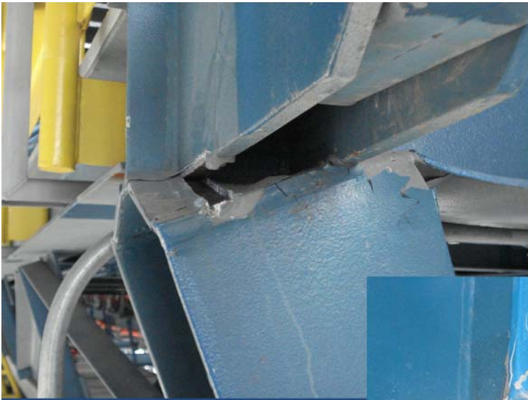
Coal Tripper Car, Coal Fired Power Station near Coronel. Failure at Moment Connections Details
