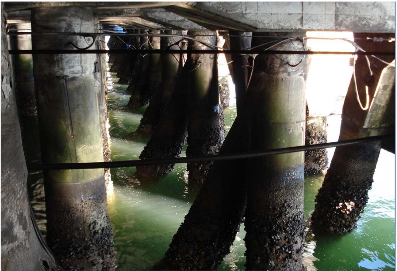
Huachipato, Vista General bajo el Muelle Pilotes Diagonales cortados., Wharf near Concepcion, Diagonal piles were sheared off at the top
